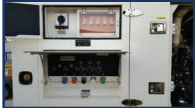
CUSTOMER CONNECTION PANEL
