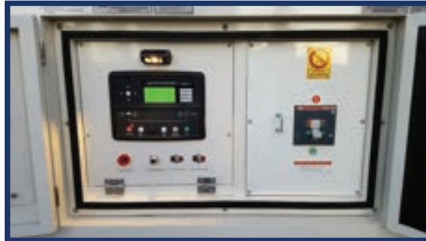
REAR CONTROL PANEL WITH MLCB
